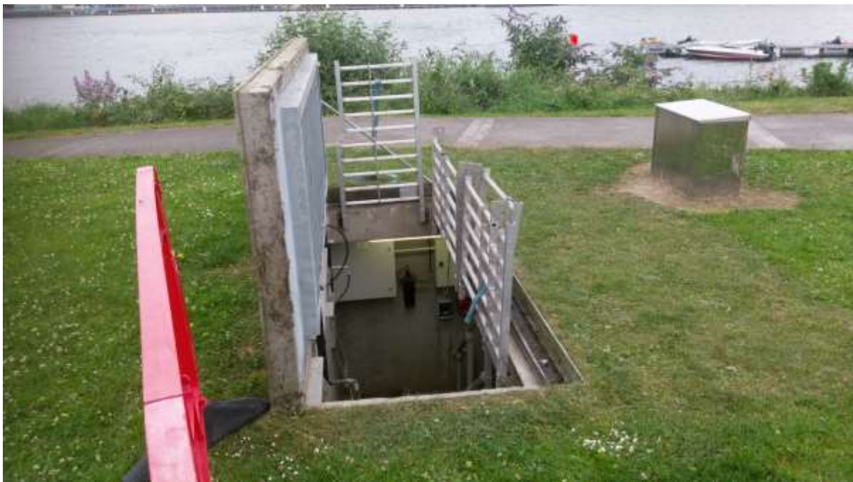
Photograph 7 Access hatch to the 2018 service tunnel shaft and gas main
